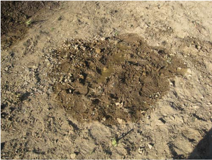
Fig. 8. The wet area at the exit of the earthwork after installation of the drainage system
